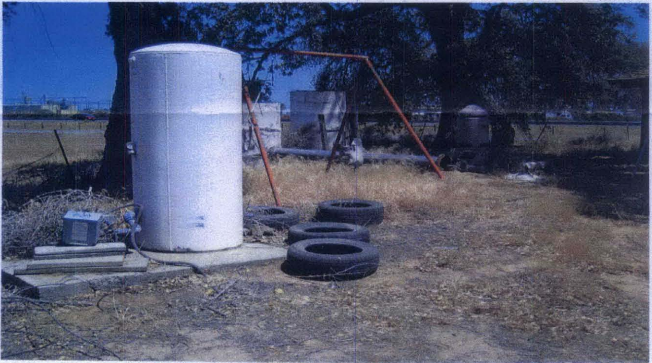
Ground water well located adjacent to single family residence.
