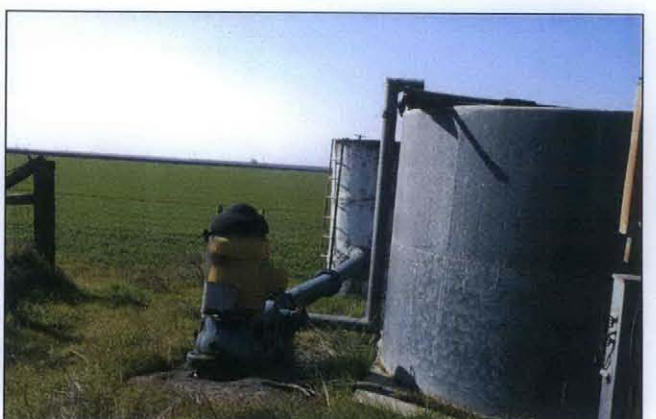
PHOTO 6: Photo of third agricultural well located on the Subject Property showing the associated tank and electrical supply box.
