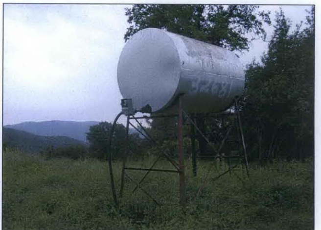
PHOTO 16: Photo showing empty 500-gallon AST located adjacent to the residence shown in Photo 8.
