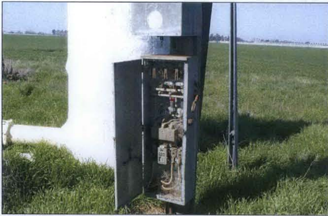
PHOTO 7: Photo showing close-up of one of the electrical supply boxes associated with one of the wells. The boxes for the other wells were similar in their design and condition.
