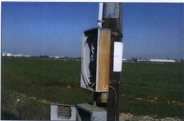
PHOTO 5: Photo showing mounted electrical supply box associated with the well pictured in photo 3.
