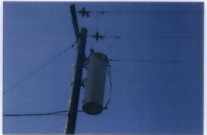
PHOTO 26: Photo showing one of the transformers mounted on one of the power lines that supply the agricultural wells on the property.
