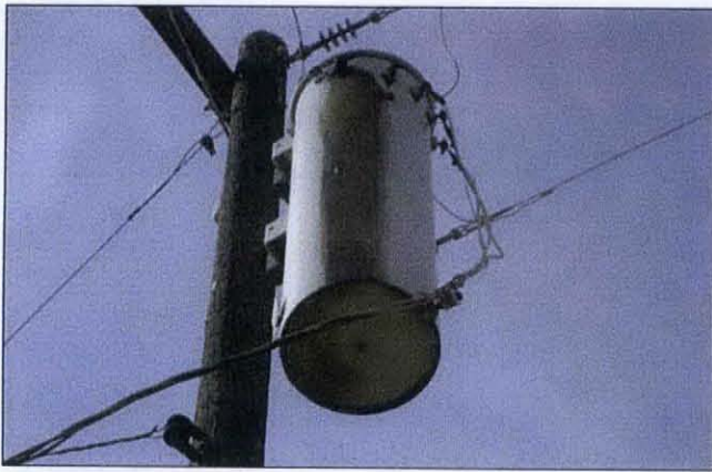
PHOTO 18: Pole mounted transformer showing signs of a potential leak.
