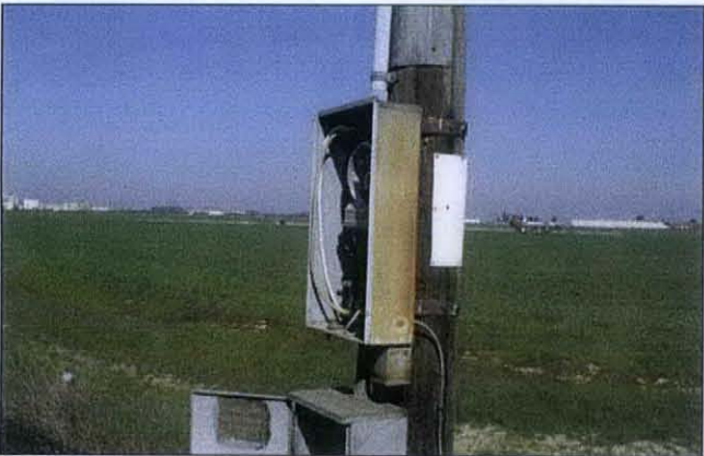
PHOTO 5: Photo showing mounted electrical supply box associated with the well in photo 4.
