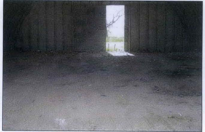
PHOTO 17: Photo showing the empty metal storage building after all materials were removed.
