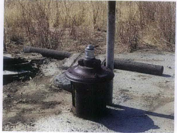
Photo 2: Photo of the well from the previous photo showing secured well cap.
