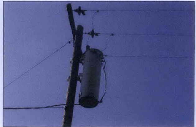
PHOTO 26: Photo showing one of the transformers mounted on one of the power lines that supply the agricultural wells on the property.
