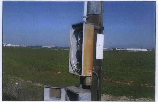
PHOTO 8: Photo showing a mounted electrical supply box associated with the well shown in photo 4.
