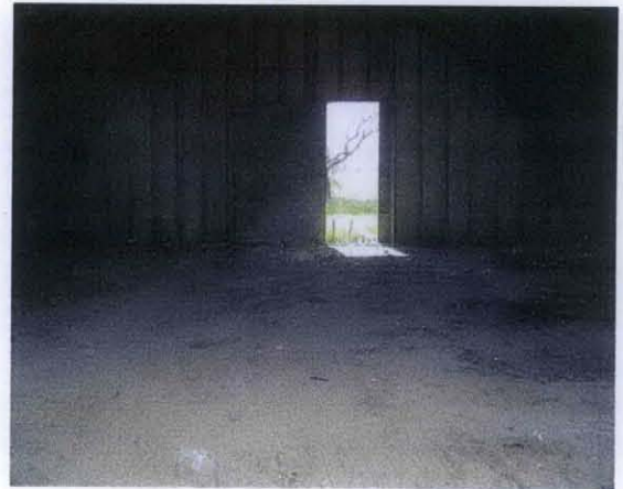
Photo 2: Storage structure from the previous photo showing cement slab and no visible surface cracks in (after clean up).
