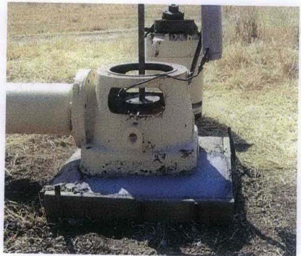
Photo 4: Photo of the well from the previous photo showing secured well cap.
