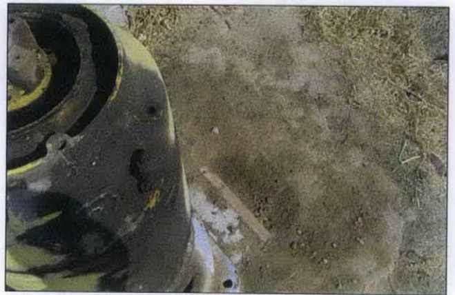
PHOTO 19: Pump motor located on one of well showing signs of hydraulic fluid leak.
